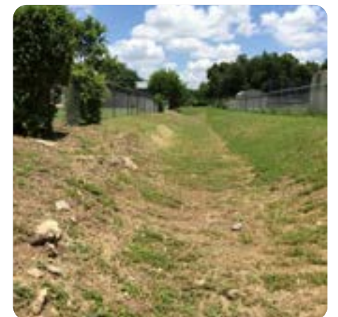
BV4: Undersized channels and culverts in the Sequoyah Subdivision from Mandan Street to Arikara Street have caused flooding to structures.
