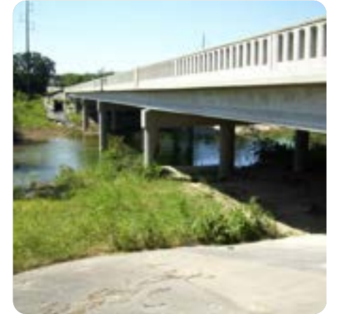
OC2: The FM 967 Bridge is over-topped by Onion Creek during a flooding event.
