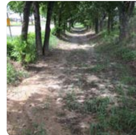
OC3: Ponding occurs along the east side of Garrison Road due to the lack of an outlet for water.
