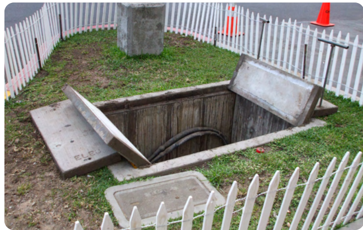
Underground Utility Vault
